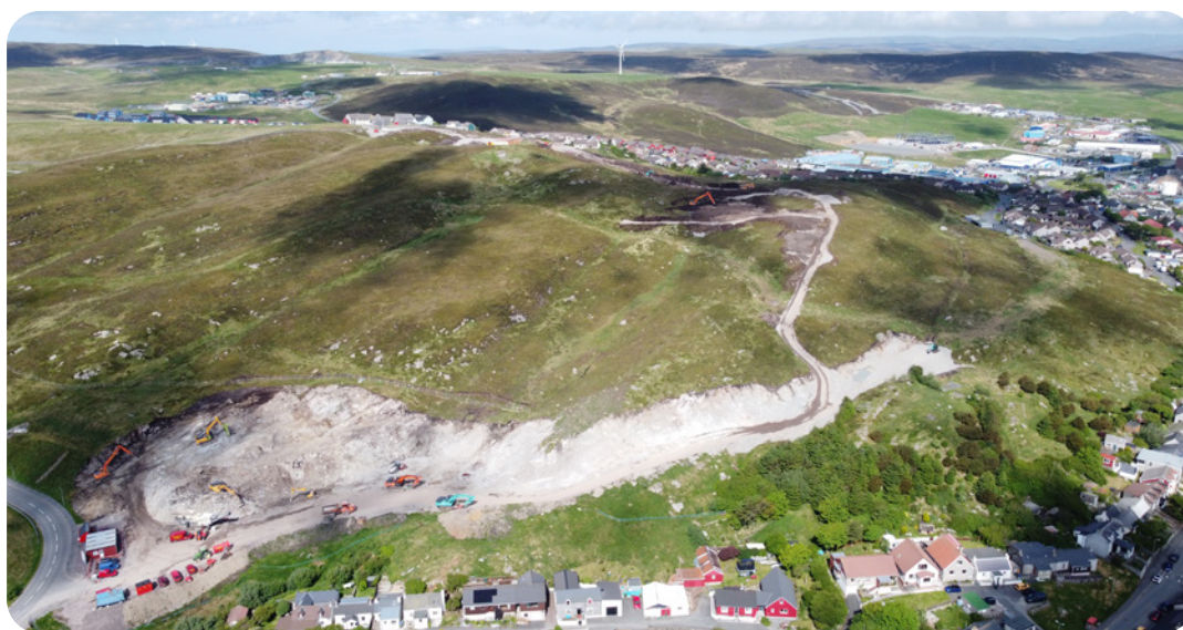
Image: North Staneyhill development site (reproduced with permission from Hjaltland Housing Association).
